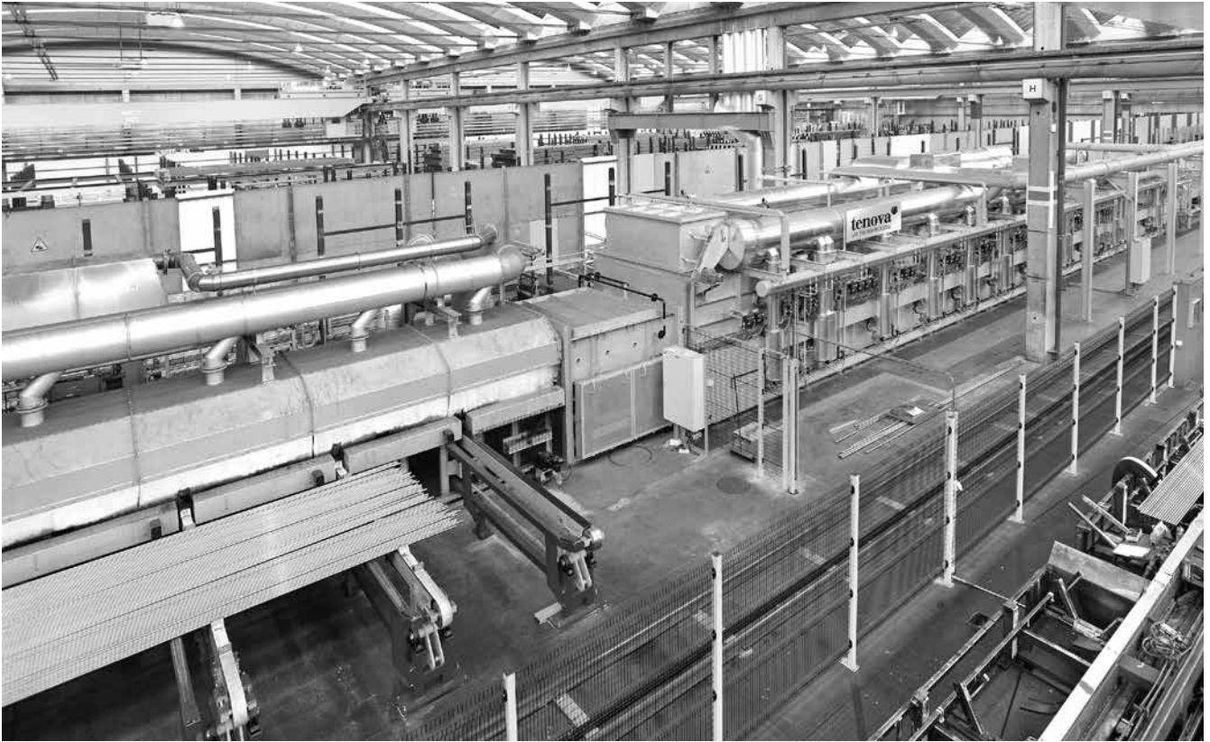
Roller Hearth Furnace for bright annealing of carbon steel tubes in a controlled atmosphere in Switzerland.
