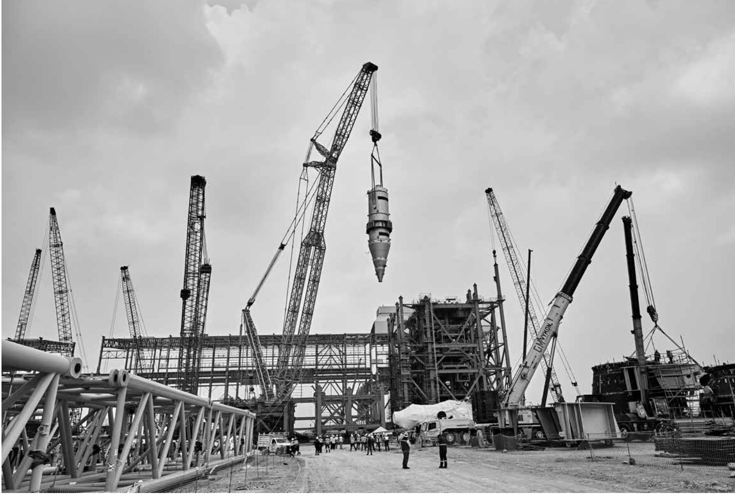
Erection of the External Cooler Vessel, ENERGIRON Direct Reduction plant at Ternium Pesquería, Mexico.
