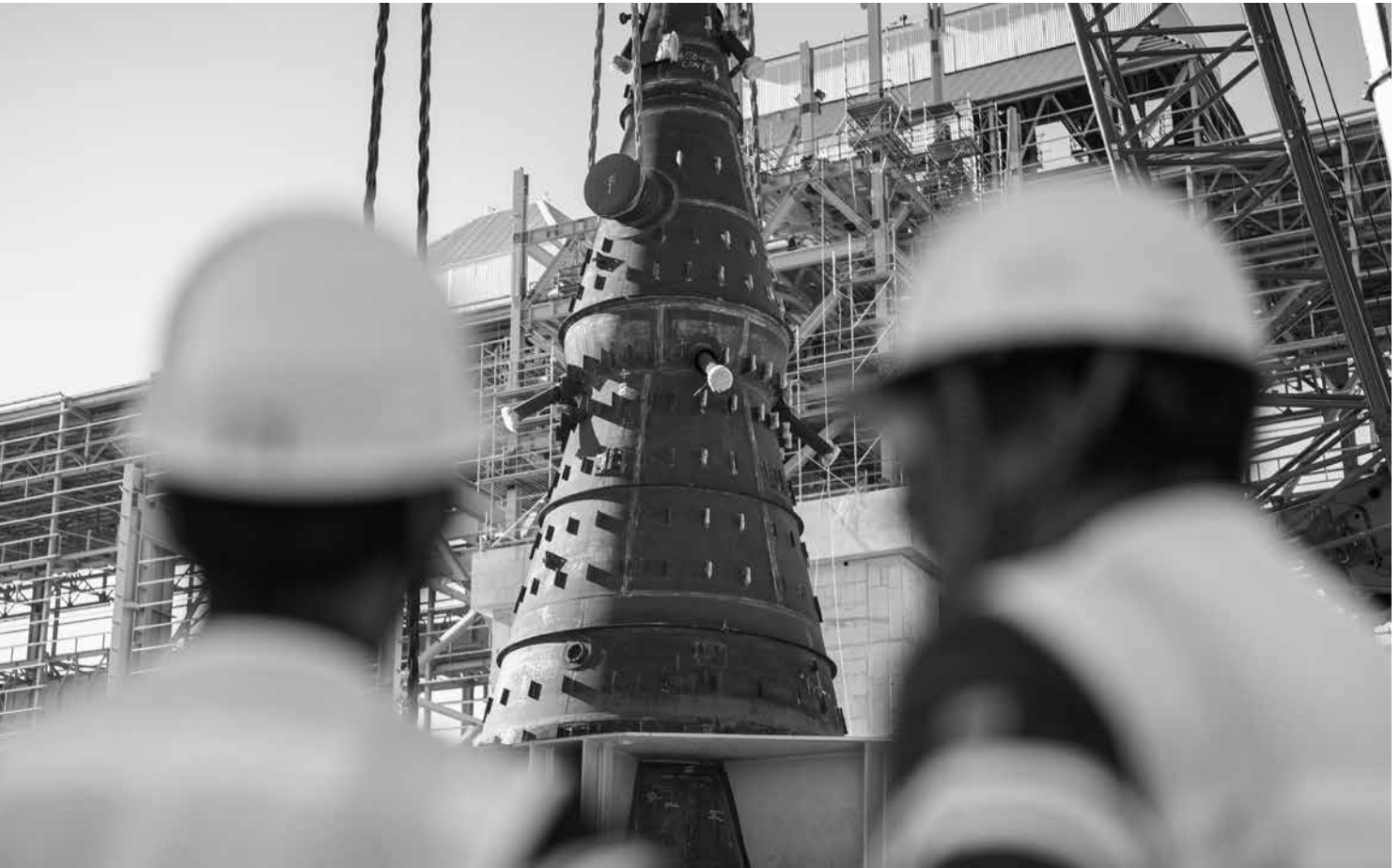
Reactor in the DRI tower, a key component in transforming iron ore into raw material at the new Pesquería steel plant.
